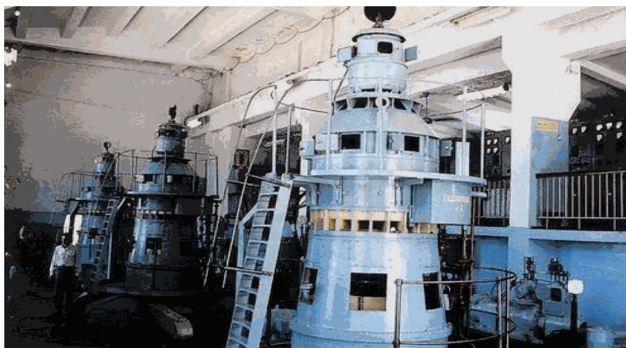
Figure 2.1. Turbine hall of the Karatal hydropower plant
