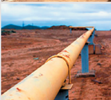
West African Gas Pipeline.
